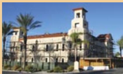
Construction for the new Casa Colina Medical Office Building began in April 2012. It is scheduled to open for patient care in early 2013.
